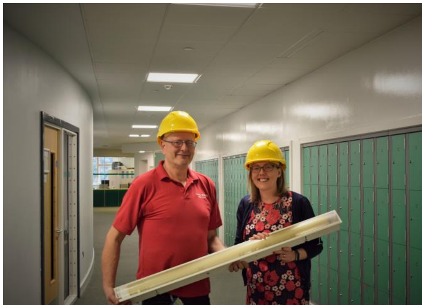
Site Manager Mr Carpenter with Mrs Elliott removing the old fluorescent lighting
